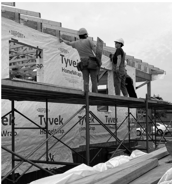
Habitat for Humanity volunteers and professional builders worked side by side on a new house.
