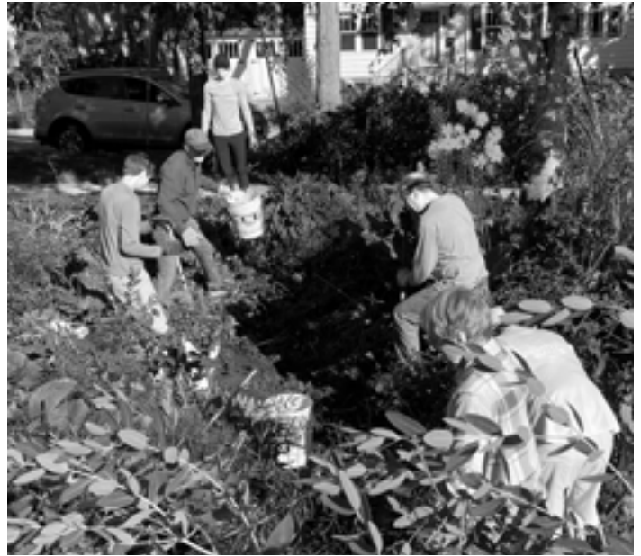
Neighborhood volunteers dug weeds and excess soil from the rain garden at Adams and Campbell streets on August 12, the first of three work days to improve the garden's function. The garden was dug down to provide more holding capacity. Later, some piping is being added to help distribute the water better, and then plants will be planted to soak up and clean the water and keep it from running straight into the lake.
