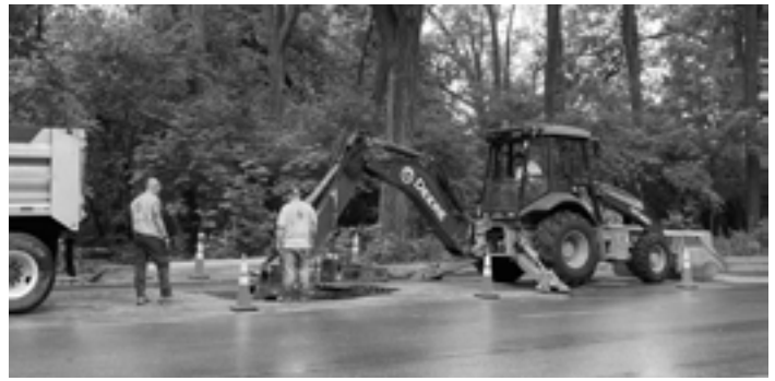
Early on Sunday, August 13, a broken water main under Drake Street spewed water and mud onto the street and nearby area of Vilas Park. Workers dug down to the broken pipe, repaired it, filled the hole and patched the pavement.
